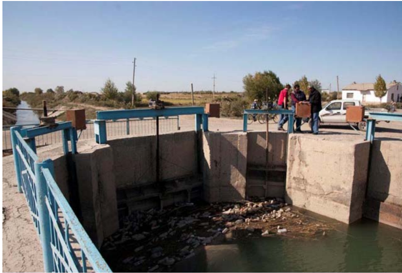
Control gates for regulating water distribution on a main canal system in Khorezm (photo courtesy of Dr. A.M. Manschadi)
